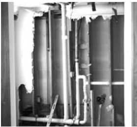
Unfortunately, as I am sure you know, when one thing needs repaired, it often means that you have to make a BIG mess to get to the problem and you end up with a BIG fix-it job.
